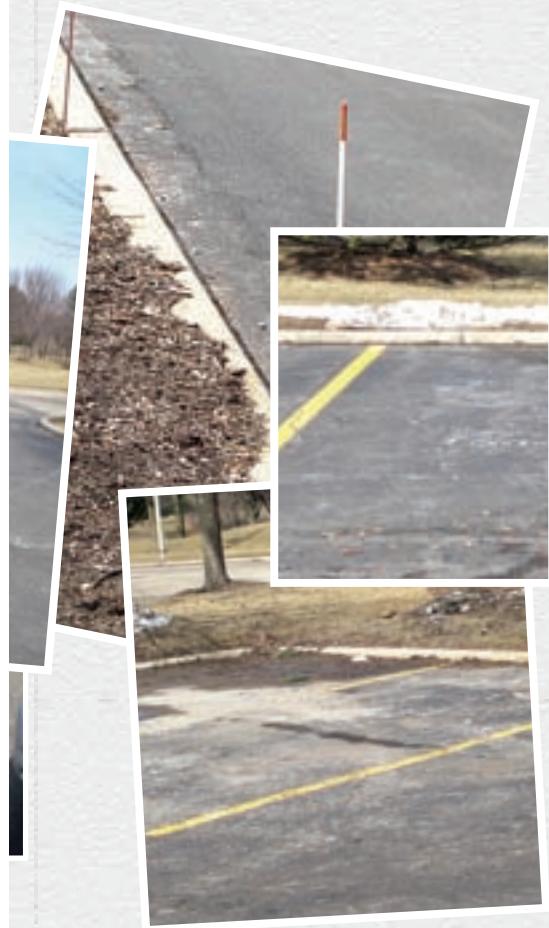
Parking stalls, curbs, overhangs, aisles and shared imperviousness contribute to oversized lots.
